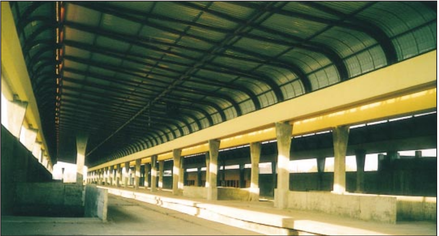
10,000 square metre of roof has been covered with stainless steel for the Airoli railway platform in Navi Mumbai.
