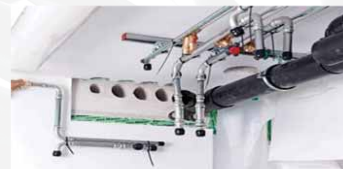
Openings for the drinking water installation realised with the Viega “Sanpress Inox” system made of stainless steel 1.4521. (Photo: Viega)
